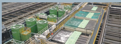
SANI launched a full-scale trial at Hong Kong's Shatin Sewage Treatment Works in the summer of 2014.
